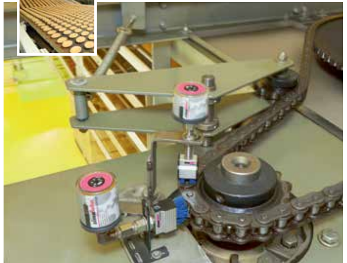
The drive chain of a transport belt, which allows rolls to cool, is cleaned with special blue brushes and lubricated with 2 simalube SL18 in 30 and 60 ml sizes.
